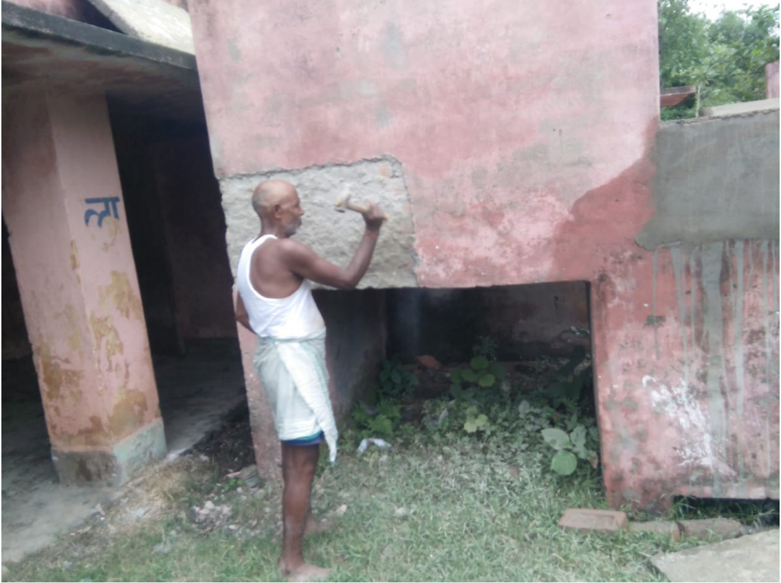
Breaking plaster because plaster is very poor
