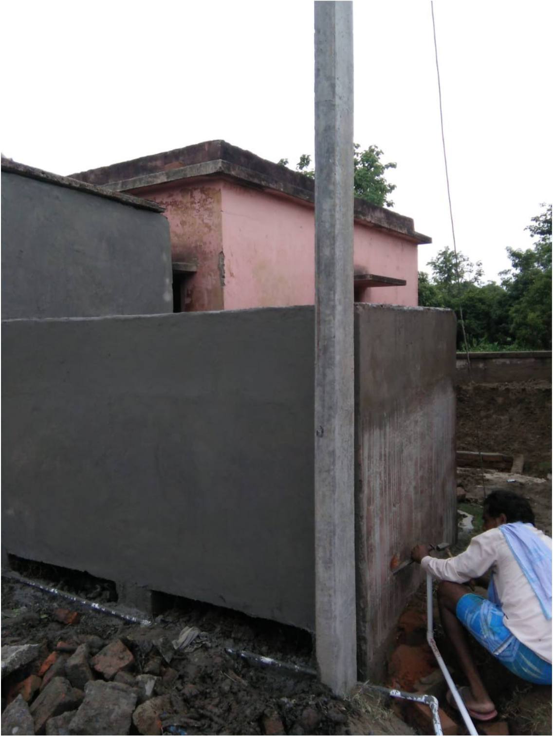
Finished water tank and fitting pipe with tank
