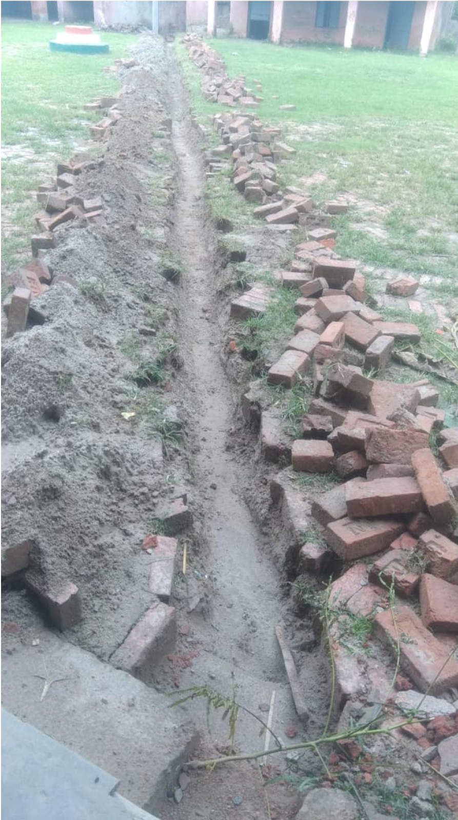
In this laid down pipeline from electric motor which is connected to tubewell and returned into again water filter Which will be near the Tubewell under the stair case.
