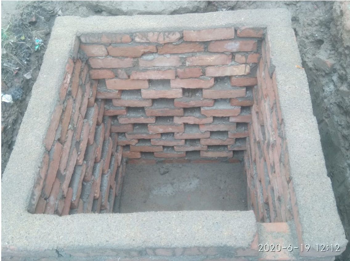
Brick work of soakpit for RWH when rain water over from tank then water will enter in soakpit by pvc pipe
